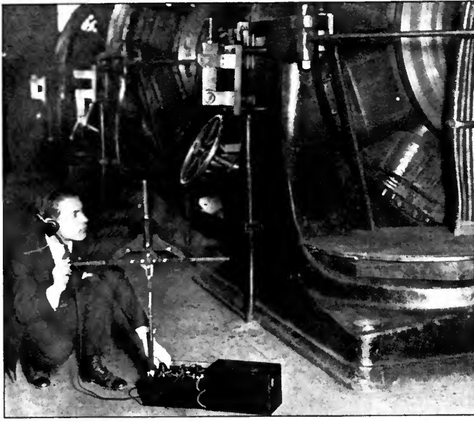
LARGE MOTORS AND GENERATORS
